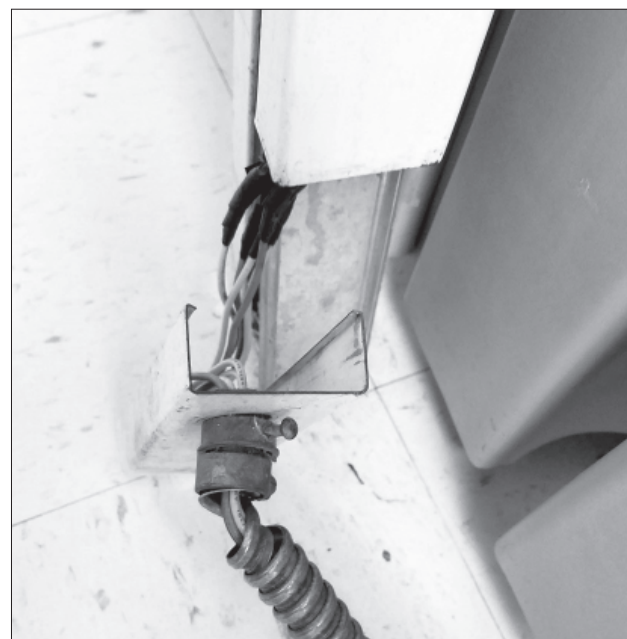
FIGURE 6–7 BROWNFIELD ISD BROKEN ELECTRICAL CONDUIT IN CAFETERIA DECEMBER 2019
