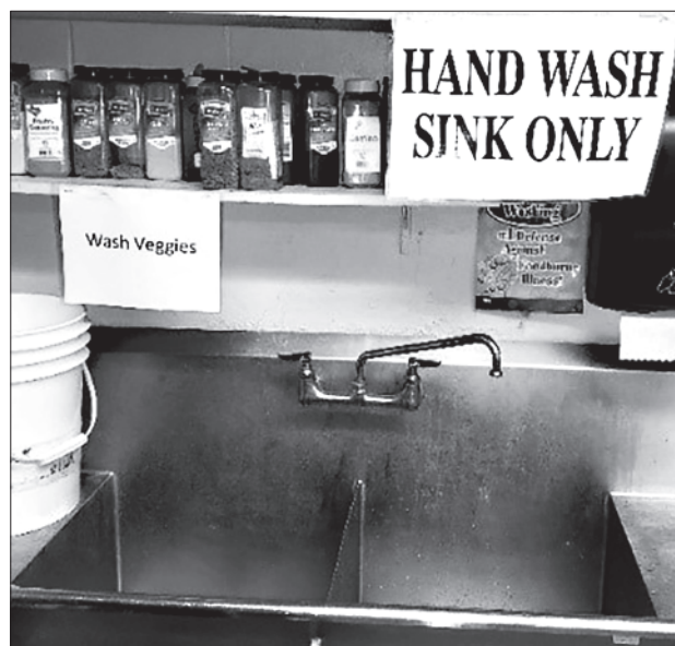
FIGURE 9–8 GONZALES ISD HIGH SCHOOL KITCHEN HANDWASHING STATION, MARCH 2020
